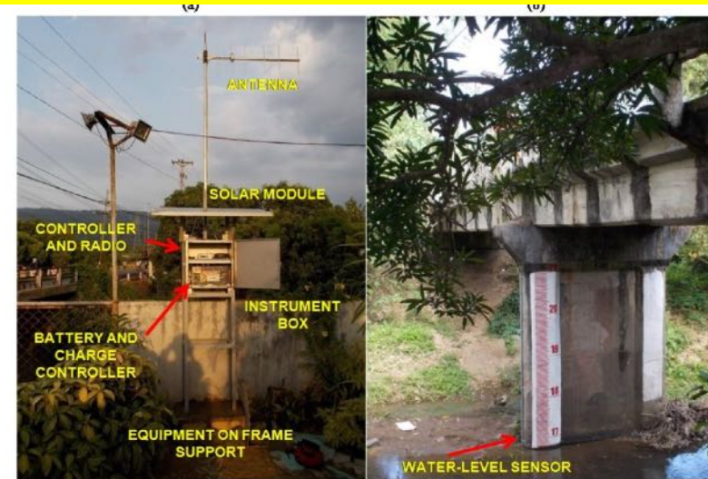
Fig. 5. Water-level Station Installation (a) on frame and (b) sensor inside a protection metal pipe bolted on bridge column.
